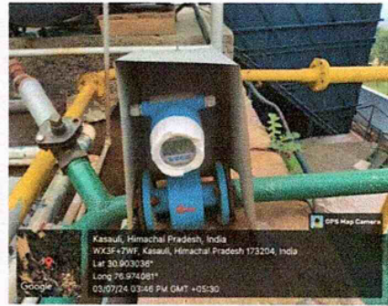
Pic No.16: Flow meter at final outlet of ETP.
