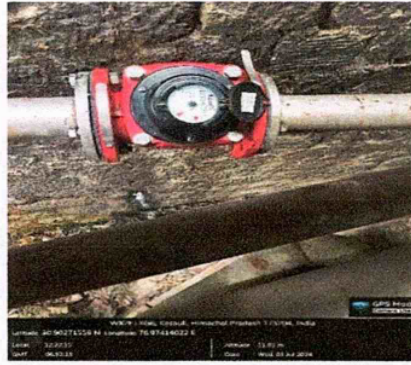
Pic. No. 13: Mechanical flow meter installed on RSW line.
