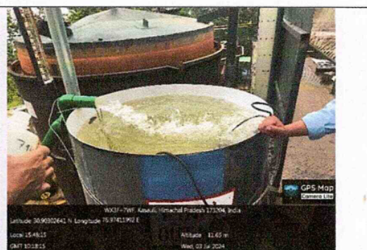
Picture No. 2: Final Outlet point of ETP near biogas holder tank (behind) of 55m 3 capacity.
