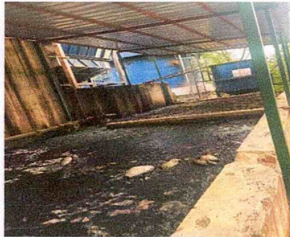
Pic. No. 15: Sludge at drying beds.
